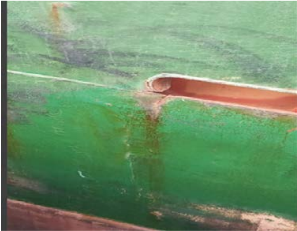
Cracked fishplate in way of freeing ports
