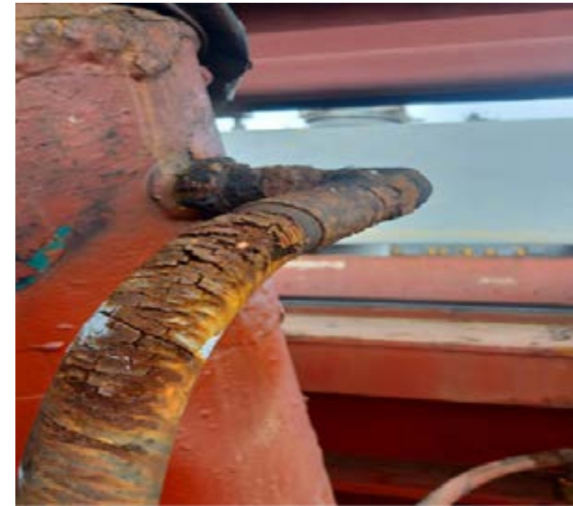
Damaged hydraulic hose
