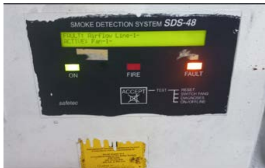
Smoke detection system fault
