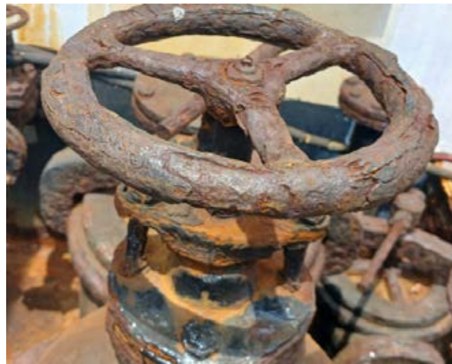
Heavily corroded valve
