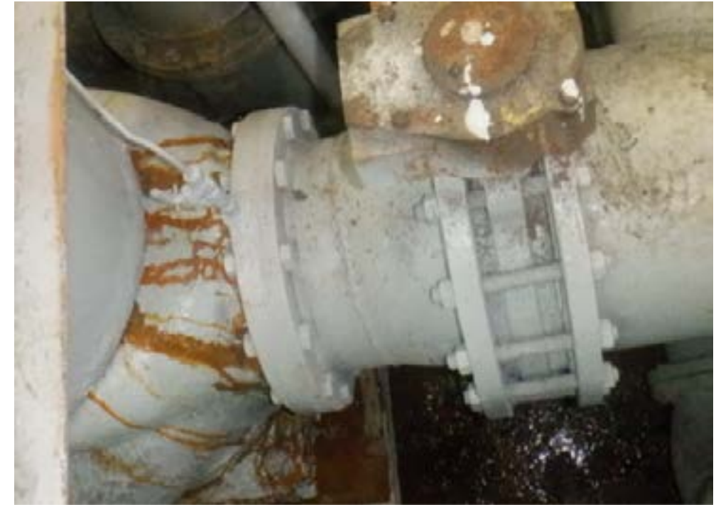
Leakage in machinery space
