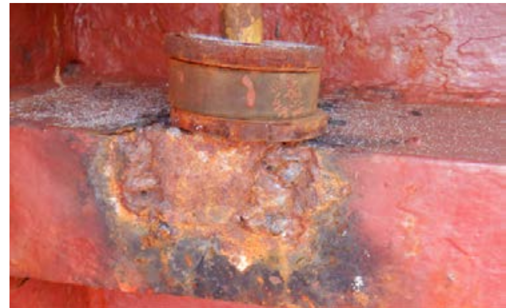
Cracked and temporarily repaired hold seal
