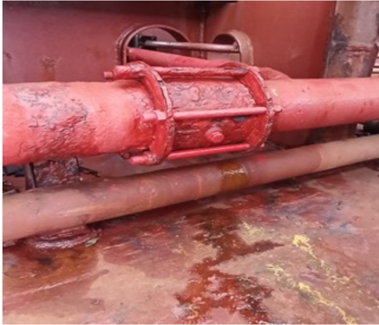
Leakage in fire line
