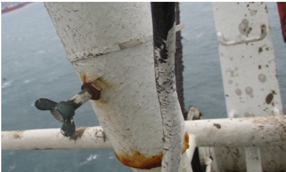
The rotating mechanism of the emergency lights is stuck in position
