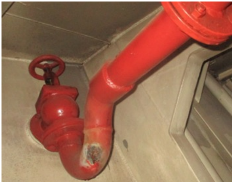
Corroded fire line
