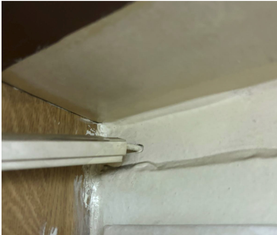
Inappropriate cable in bulkhead penetration
