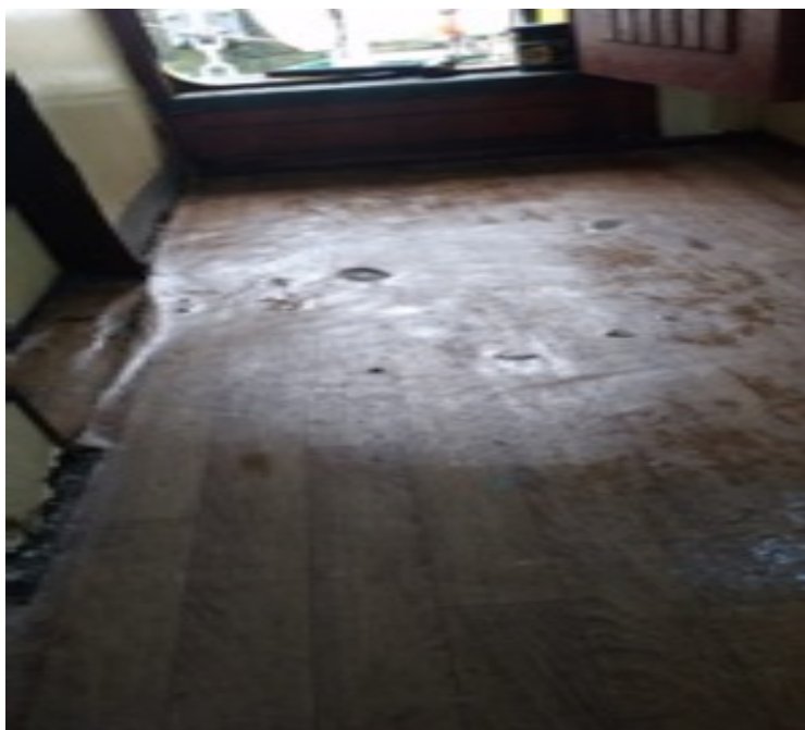
Floor covering partly worn out
