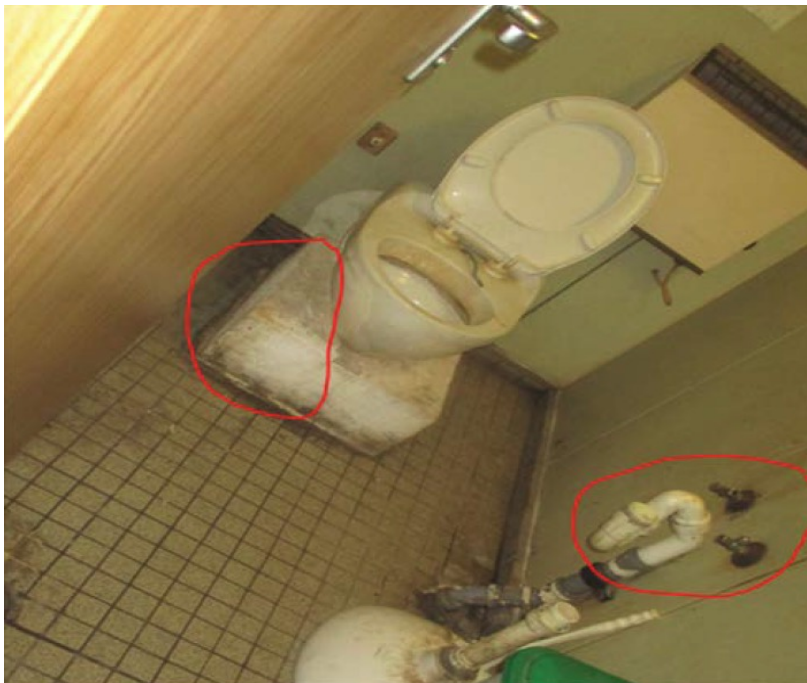
Improper condition of toilets
