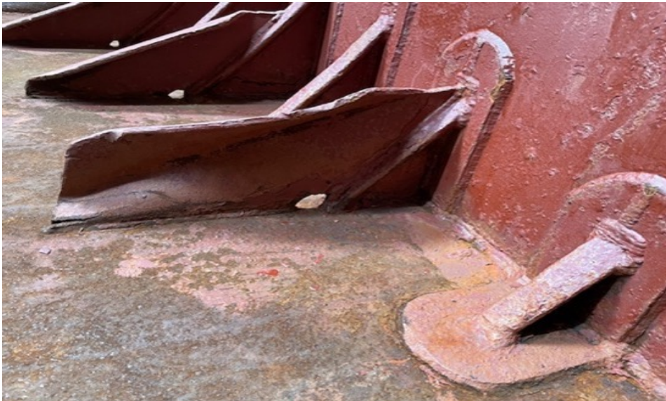
Damaged bracket in cargo hold
